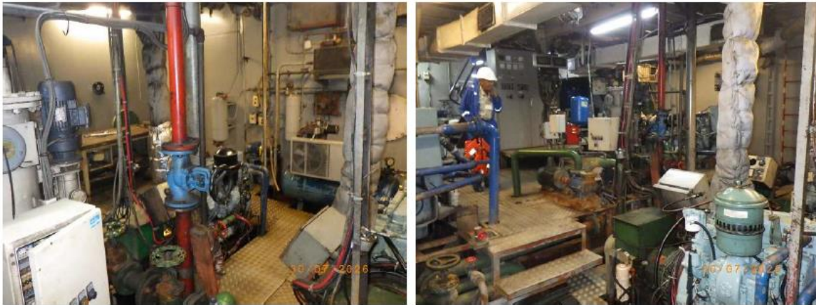
Overview Engine room with main engines and generators
